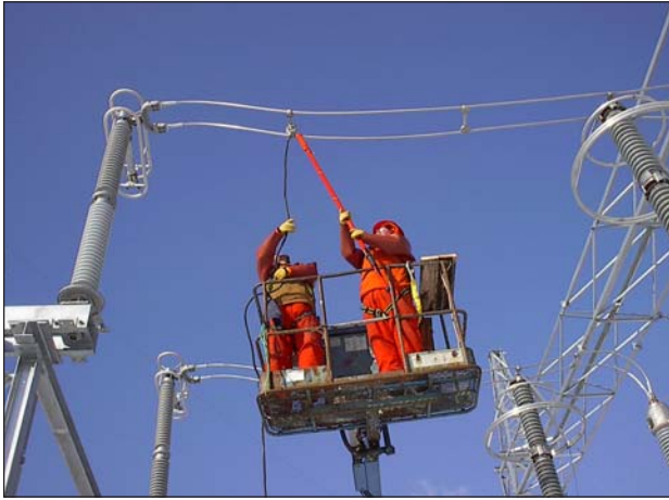
JL Dave Giannotta & JL Danny Brooks placing grounds on 345KV BUSS in substation in Rochester, NY.
