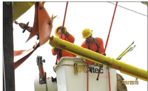
LU 1249 34 Kv Hot Sticking LaFayette, NY Harlan Electric. A6 Ben Murphy and JL Grant Bucktooth
