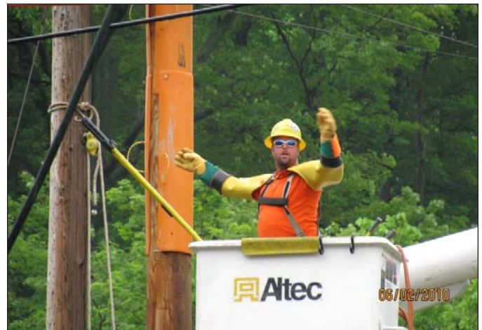
JL Tim Daley, Cazenovia Substation Harlan Electric
